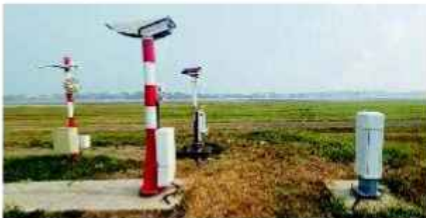
Fig. 4.17: Automated Weather Observing System installed at Mumbai Airport.
