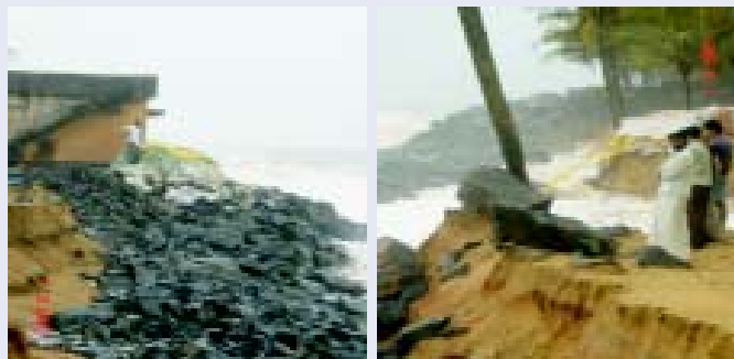
Loss of beach and damage to dwelling house due to high wave activities
