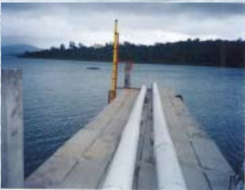
Acoustic Tide Gauge installed at Minnie Bay
