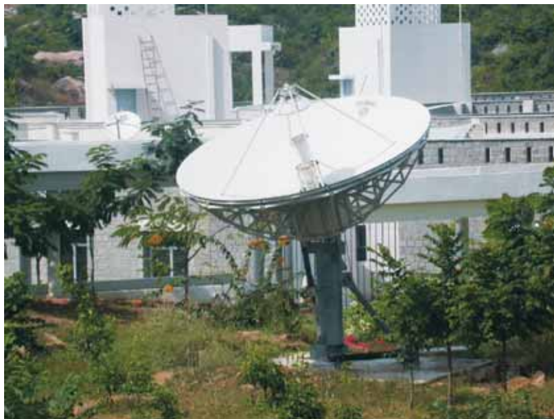
Communication facilities to receive data from seismic stations, tide gauges and BPRs in real-time
